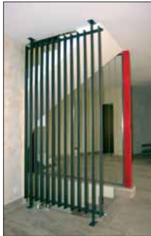
Bild 3. Der Radiator im Treppenhaus, geregelt über einen KNX Ventiltrieb Figure 3. The radiator of the staircase is controlled by a KNX valve and also functions as a handrail.
